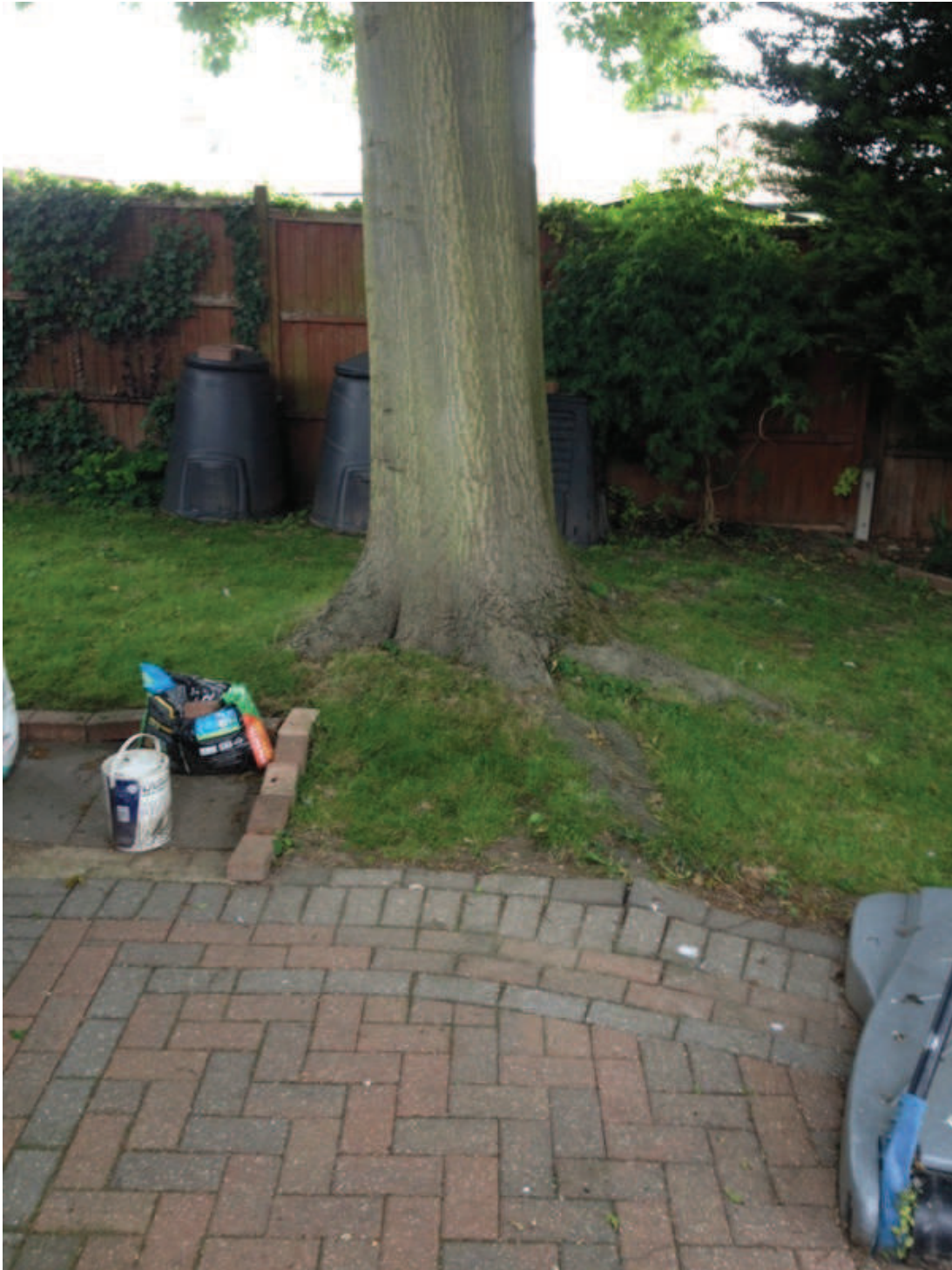
Figure 6: The localised root damage to part of the block paved patio
